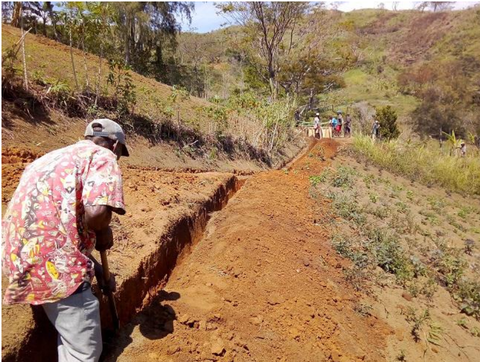
Around 7 km of trench was dug by hand to contain the pipes
