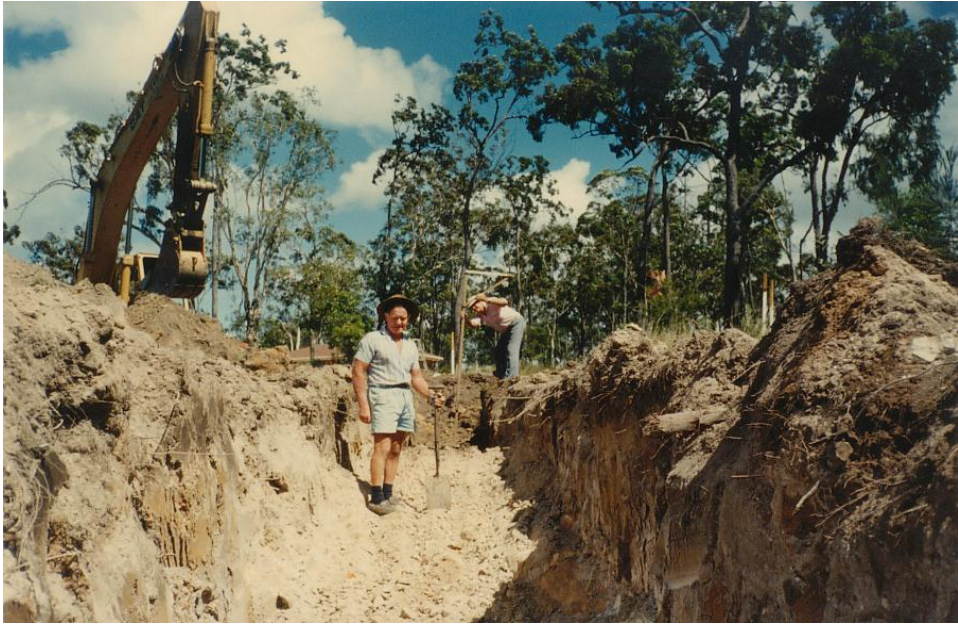
Sewerage trenches at Shaftesbury Campus. Much of our work will never be seen.
